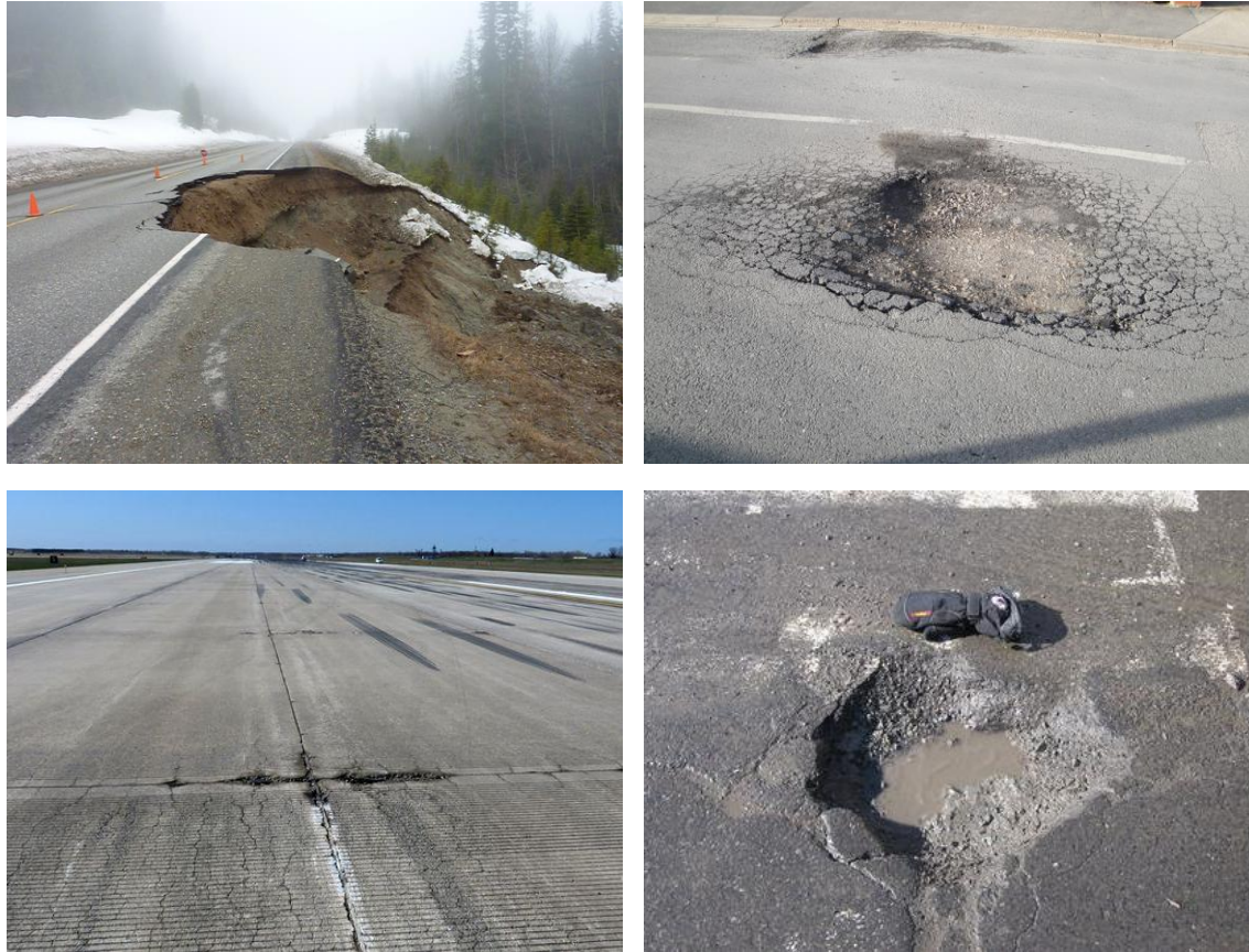
Moisture-related pavement distress and damage
