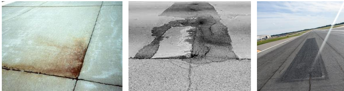
Moisture-related pavement distress and damage
